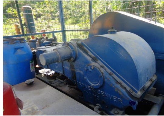
BC 881522-bomba Gardner Denver FDFXDH
